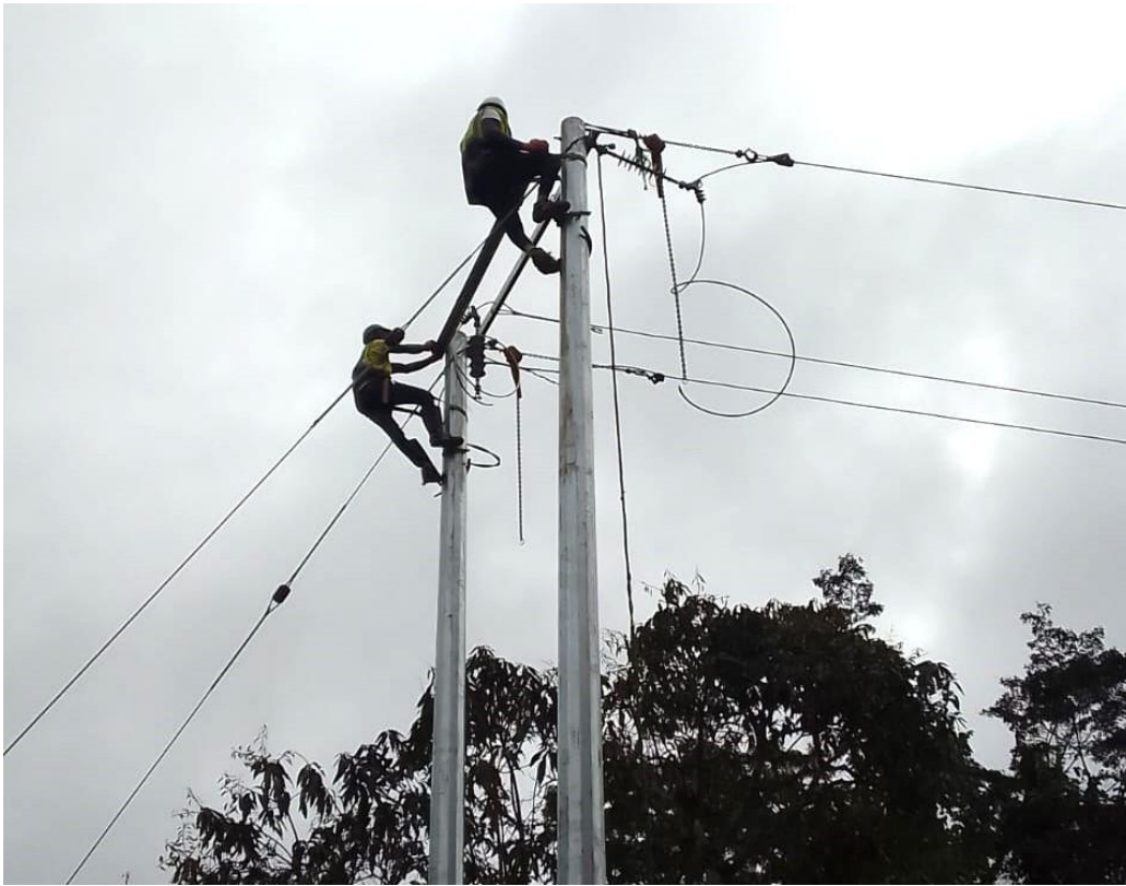
Figure 7: Contractor replacing bare conductors with insulated cable — Johnny's Town, Voinjama District, September 2024
