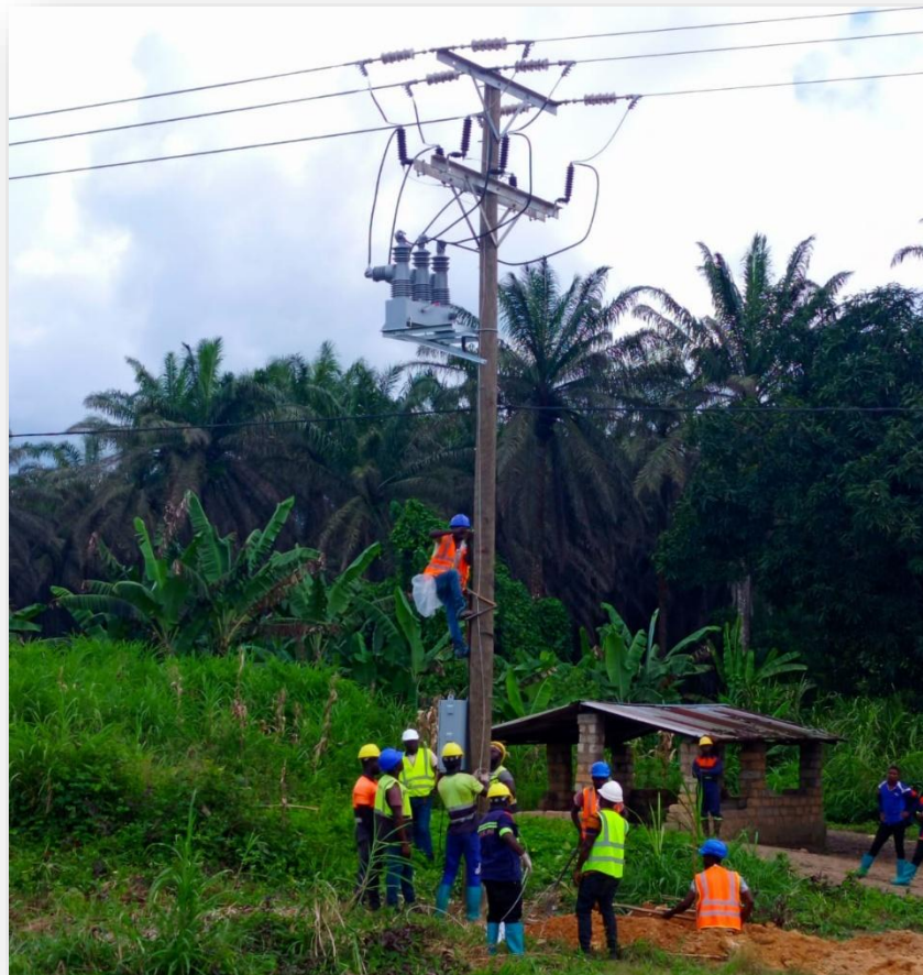
Figure 2: Pole-mounted distribution transformer installation, Veseli, Voinjama District
